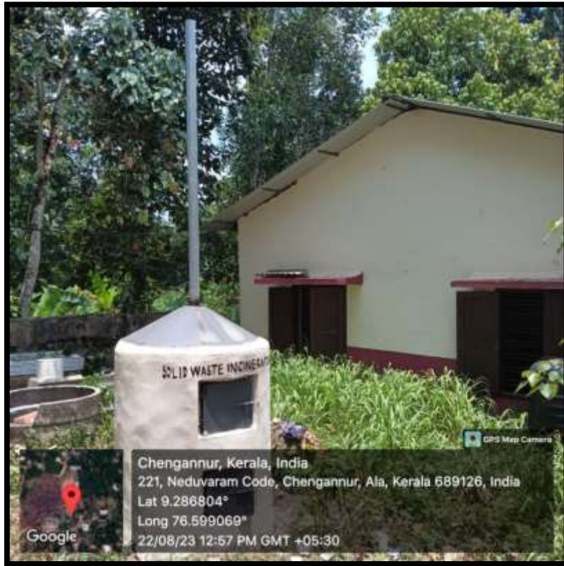
Solid Waste Incinerator installed at the campus
