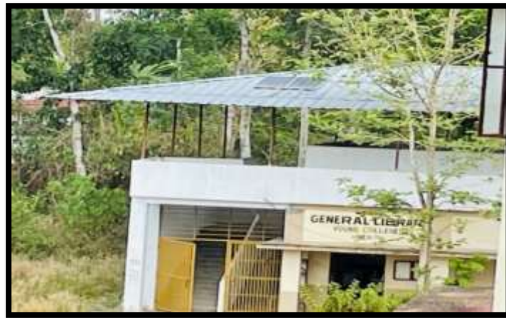
Solar Panel installed at the college
