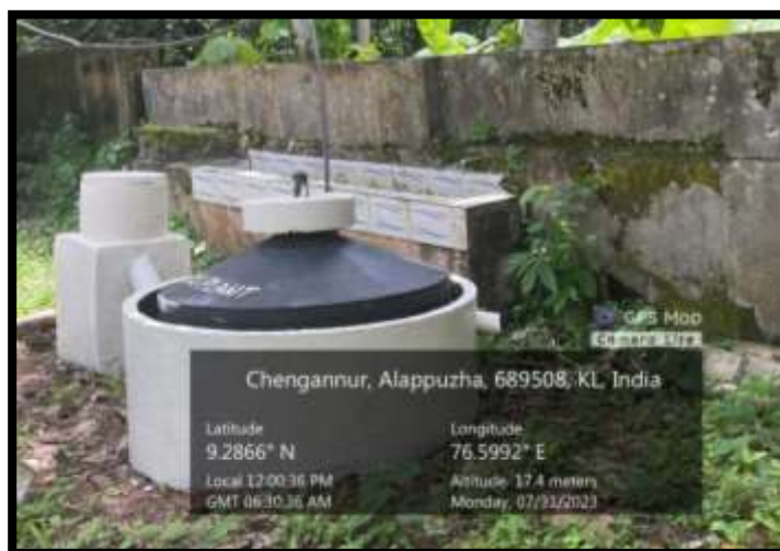
Biogas Plant at the Campus
