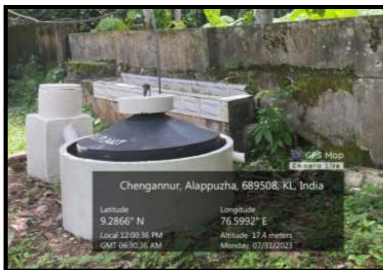
Biogas Plant at the Campus
