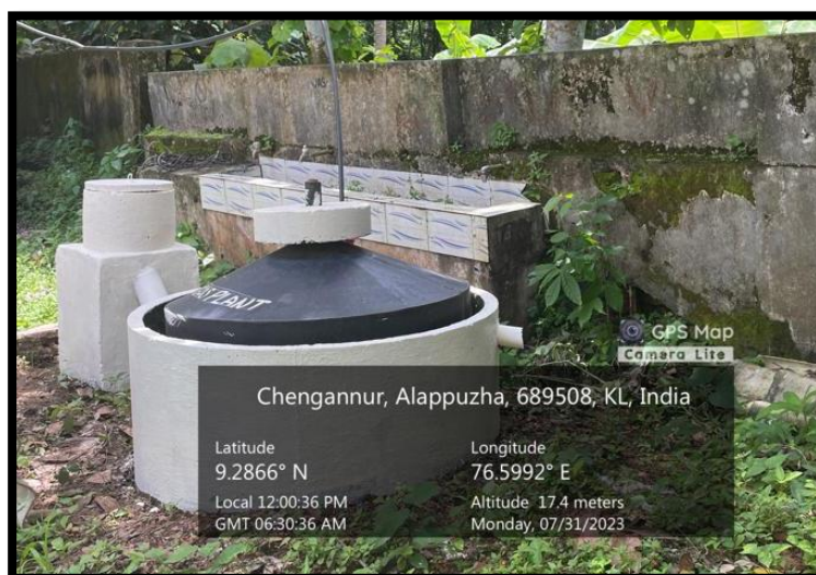
Biogas Plant at the Campus
