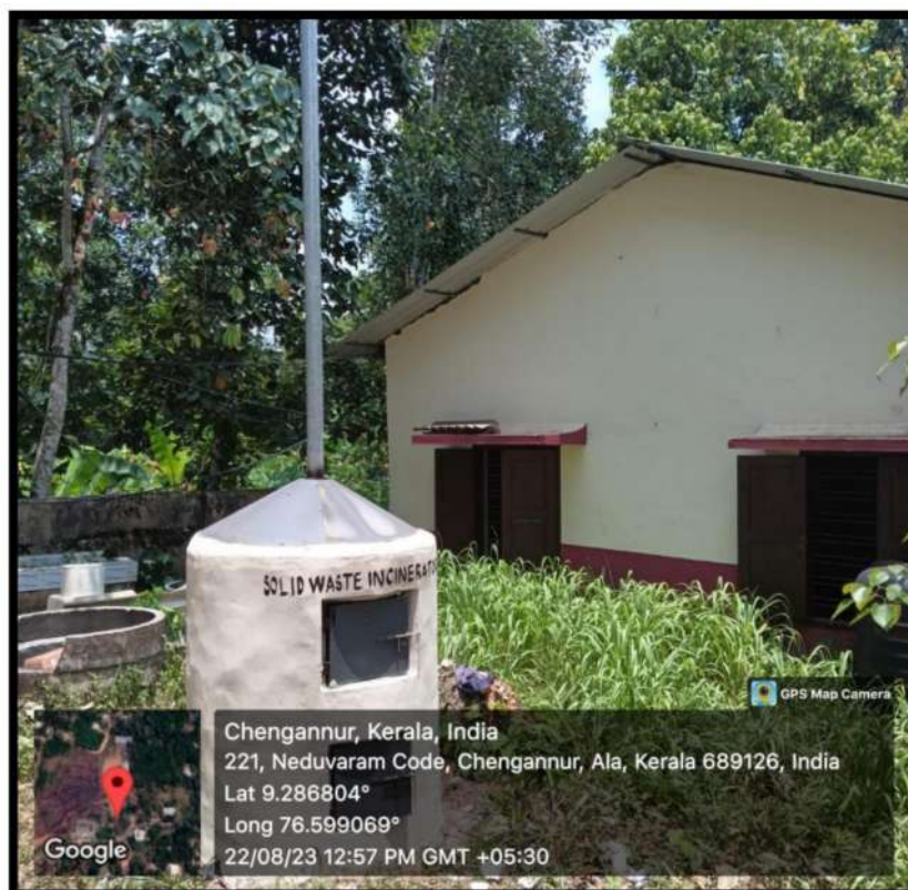
Solid Waste Incinerator installed at the campus
