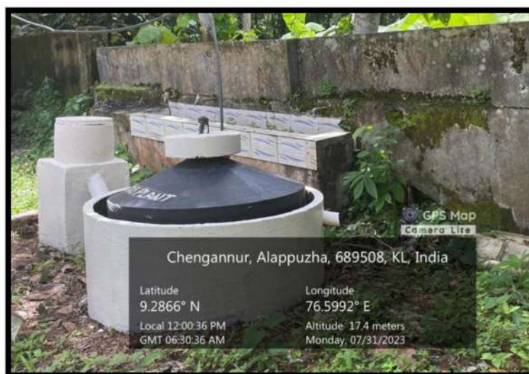
Biogas Plant at the Campus
