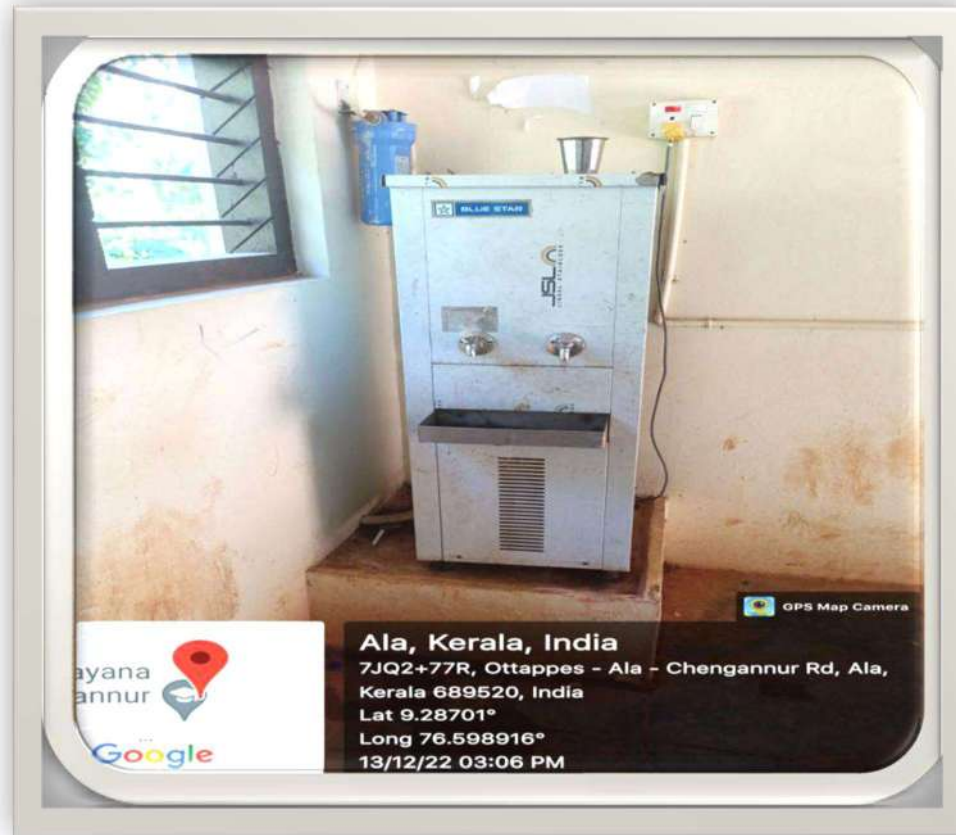
Drinking/Purified water facility
