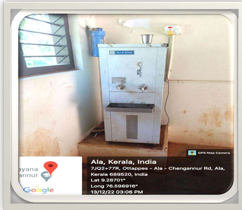
Drinking/Purified water facility
