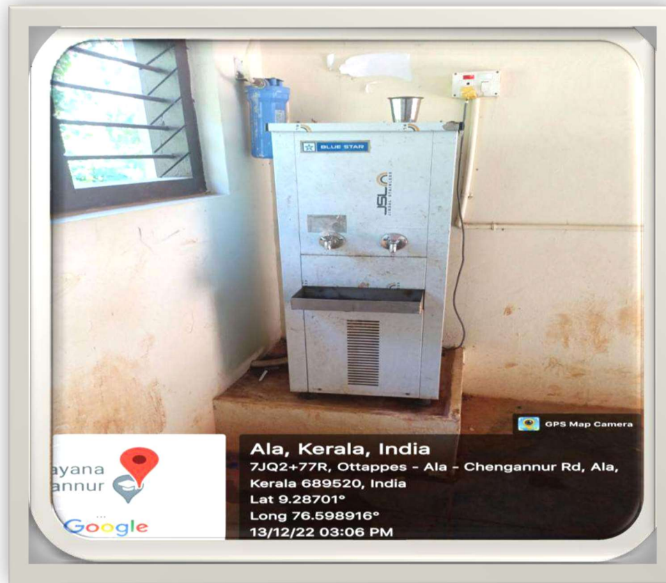
Drinking/Purified water facility
